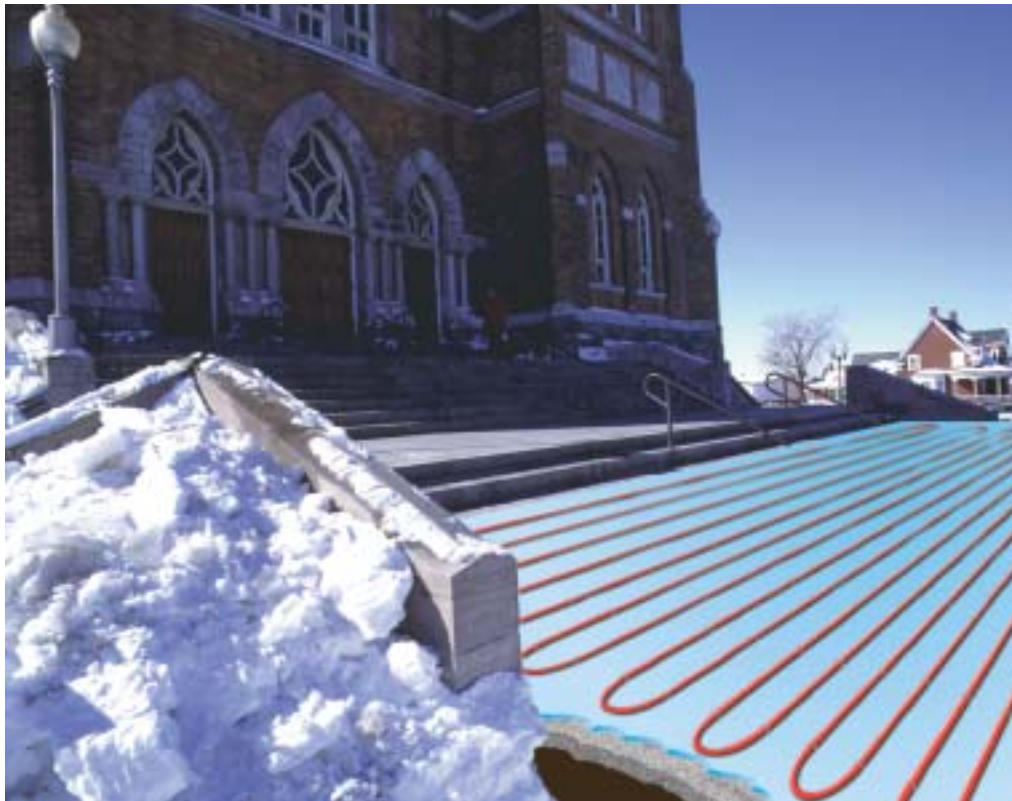
Coiled beneath the entrance to this church, a RAUPEX SIM system keeps the walkway free of hazardous ice and snow.
